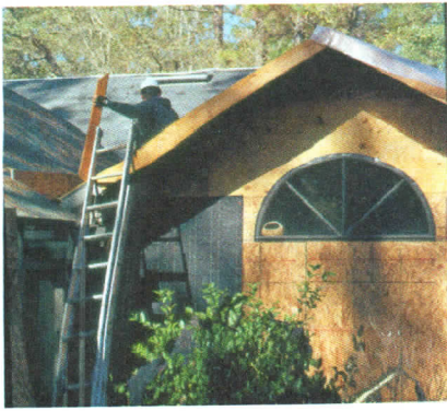
The roof is the most important element of the home. Use rated roofing material.
